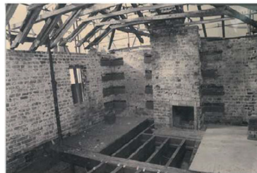
Record photo from 1990. First floor, north and west walls showing elbow ties
