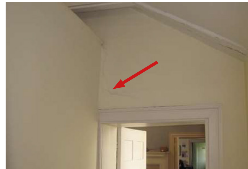
8. Upper ground floor; crack to finishes
