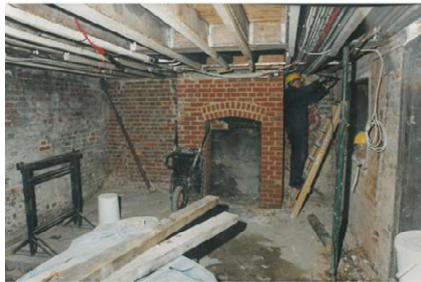
Undated record photo (assumed 1990) at ground floor, north wall, showing work to first floor joists
